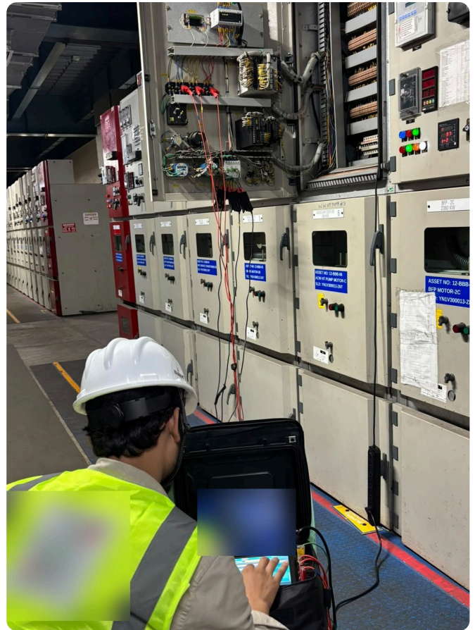
Motor condition monitoring.
