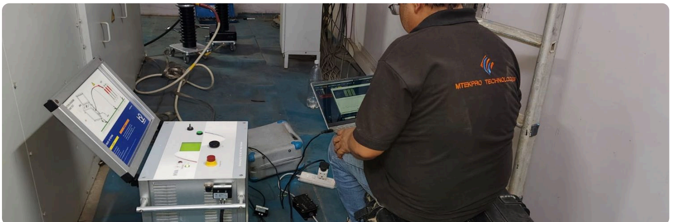
VLF testing in progress — MTEKPRO engineer on a client site.
