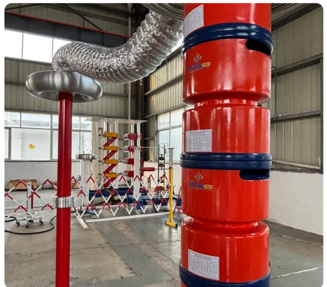
Series resonant test set for onsite HV testing.
